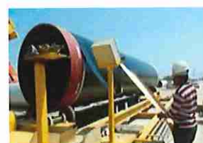
North Ezzor Water Station Water Pipes
