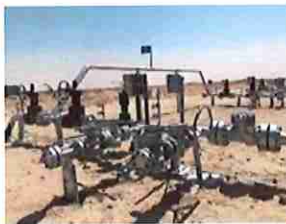
Oil Well Production Lines
